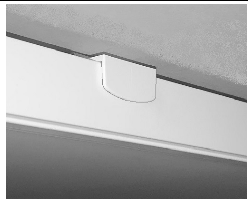
Figure 5. Properly installed clip.
